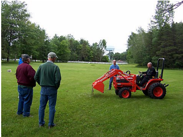
W8DXX's tractor not only drove the generator, but also helped get some of those tower anchors out of the ground.
